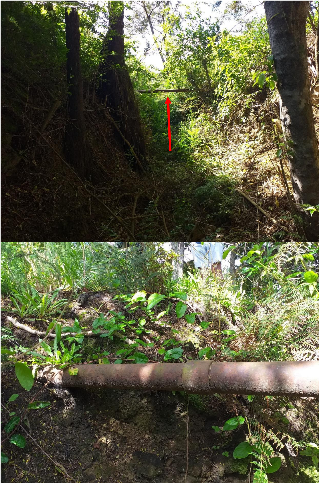
Figure 46. The waterpipes crossing the tramway cutting, just below modern overburden and stratigraphically later than the tramway cutting itself.
